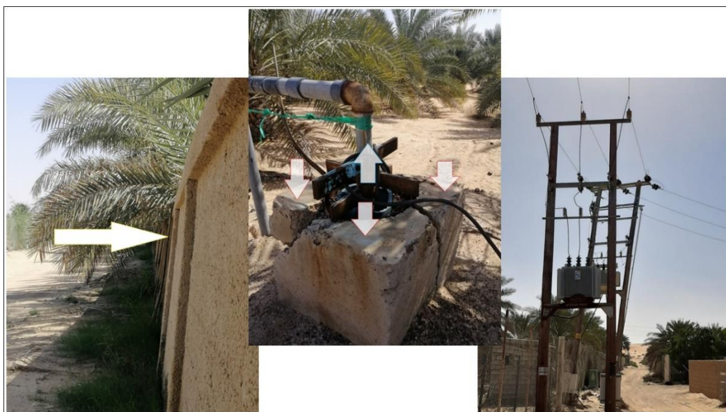
Figure 2 Land surface subsidence evidences. On the left the leaning wall, at the middle the protrusion well casing, and on the left the leaning of electrical pillars.
