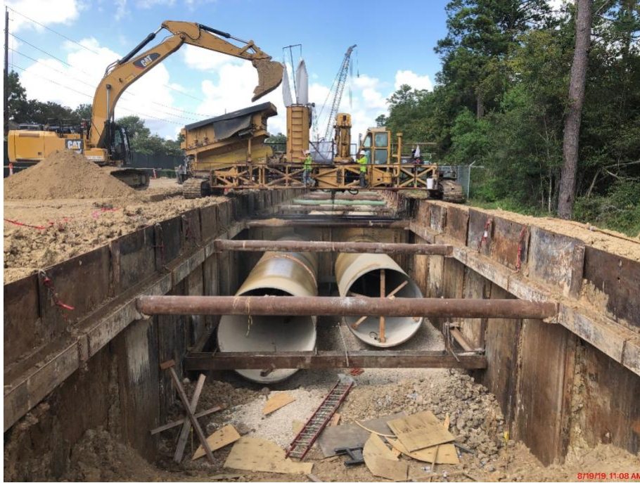
Figure 4 (main) Photo of construction of dual 2.74-meter raw water lines from Lake Houston to the Northeast Water Purification Plant (courtesy Steve Berckenhoff); (inset) Subsidence District officials near raw water pipeline (courtesy Harris-Galveston Subsidence District).
