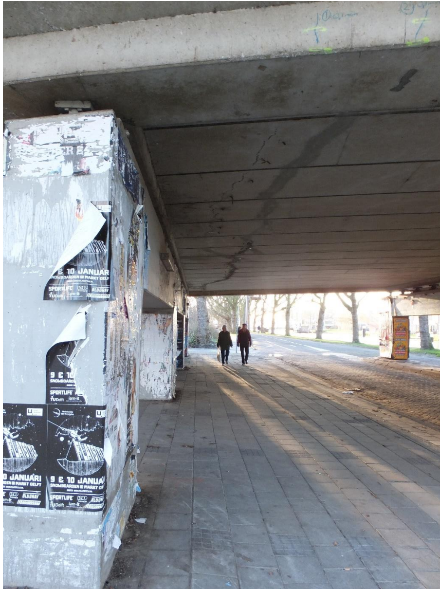
Fig. 2. Example of cracks in the concrete
